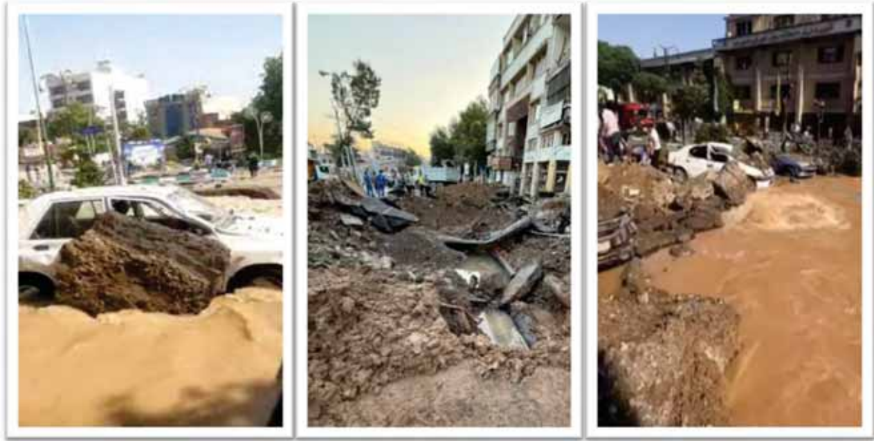
Targeting of main water pipeline led to flooding in Tajrish neighborhood
